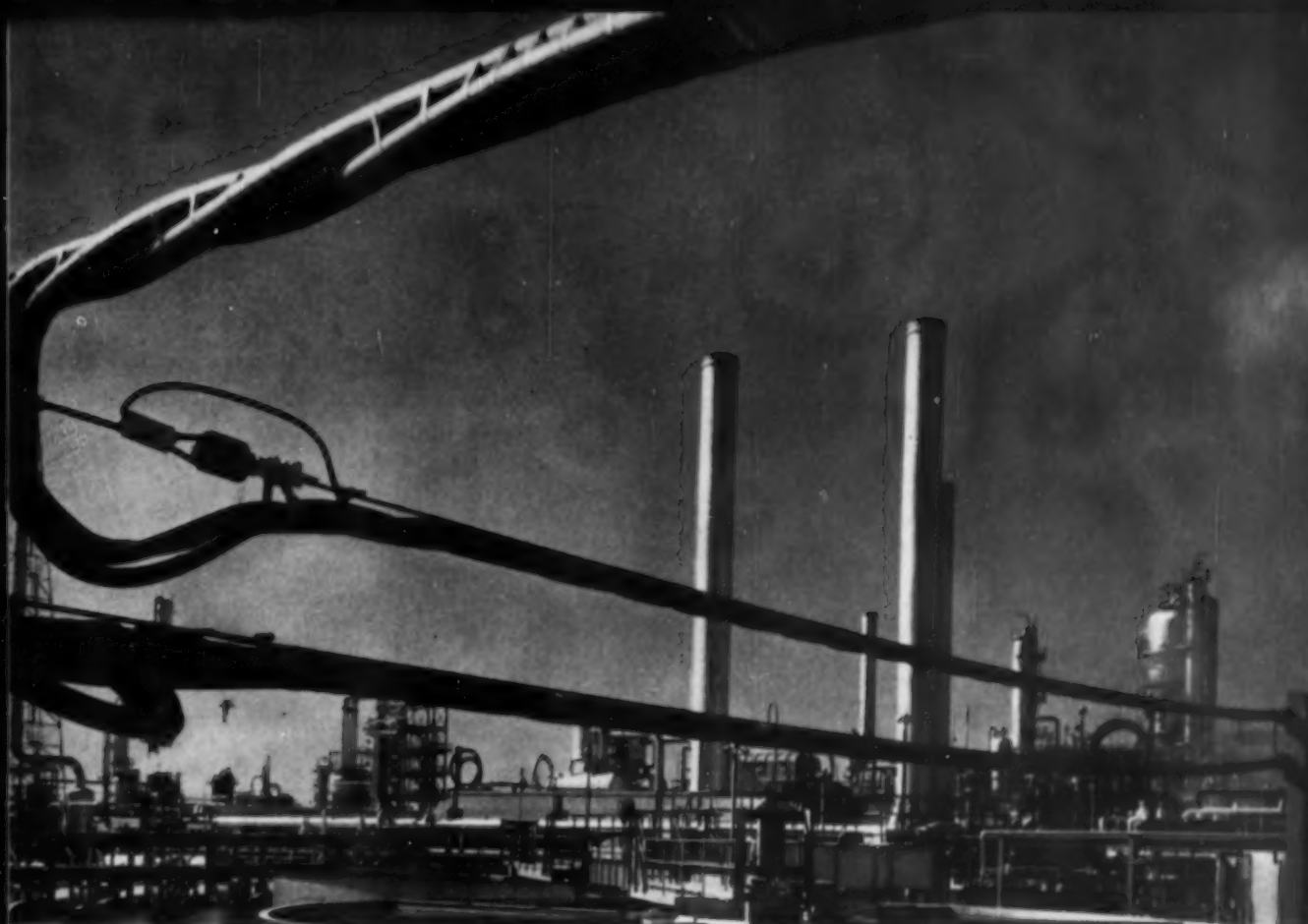
Anaconda 15 kv aerial cable installed at oil refinery.
